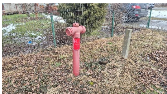
7. Hydrant – direction NE
