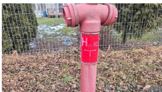
8. Hydrant – direction N
